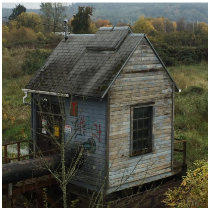
Old Pump – 1940s
