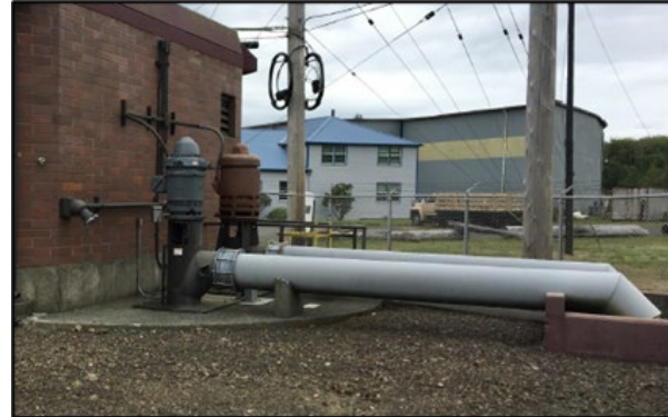
Pic 8 -- Queen Ave. Pump Station
