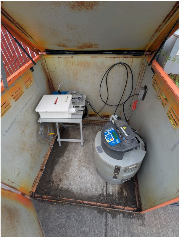
Autosampler and datalogger inside enclosure
