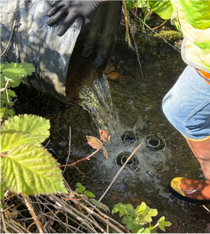
Sediment traps located at outflow
