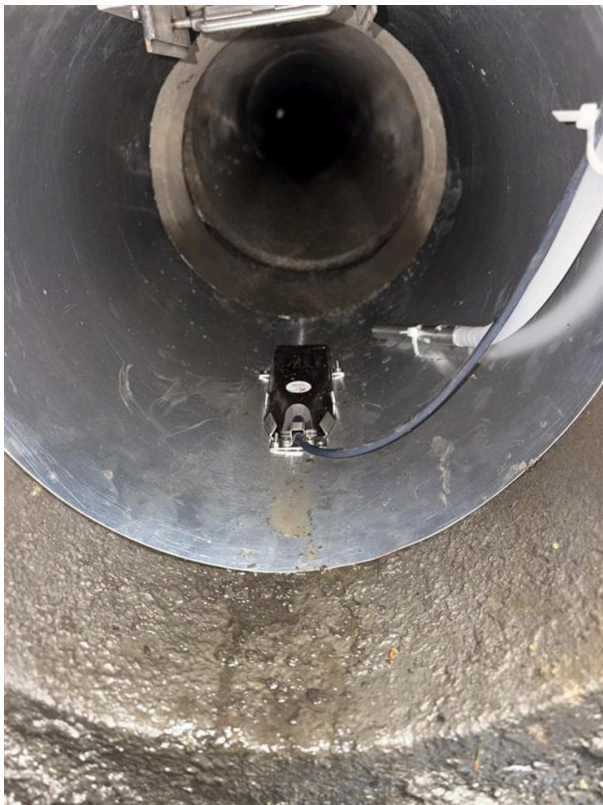
Close-up photo of flowmeter
