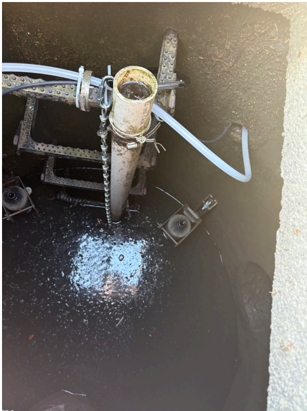
The pressure transducer is hose-clamped to a brick for weight, placed in the sump, and secured by chaining it to the ladder for stability. This photo shows the chain attachment
