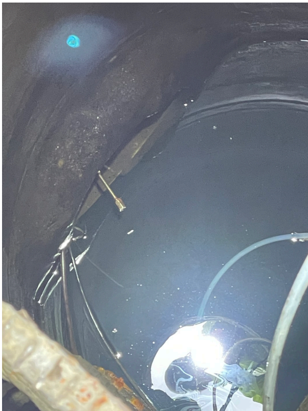
AV sensor located in pipe to the left of the sump.
