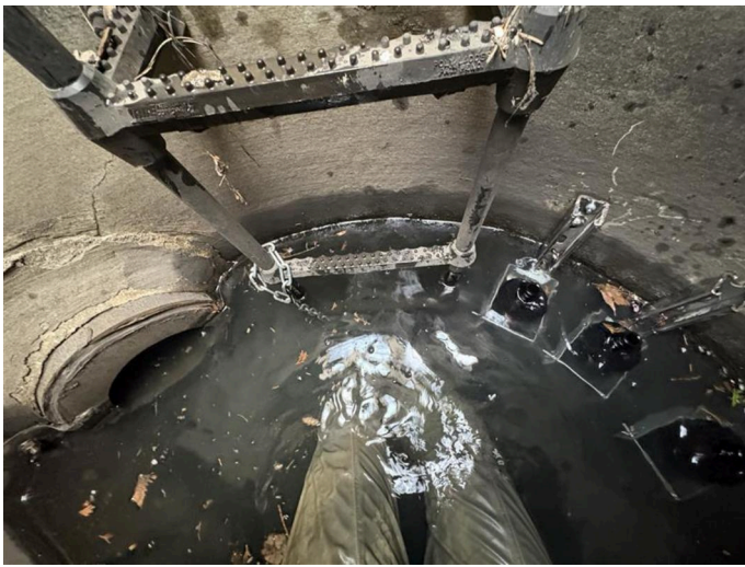
Pressure transducer is attached to the ladder by a chain and located below the water's surface
