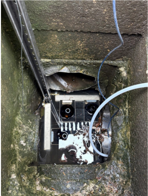
Bird-eye view of sediment traps in the sump of catchbasin (CB)
