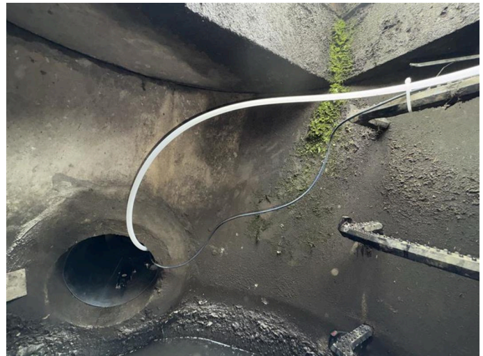
Intake tubing and flowmeter cable inside CB
