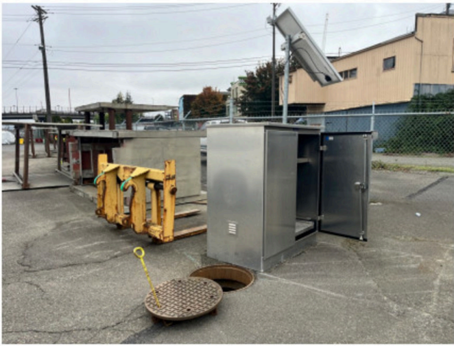
Monitoring equipment enclosure.
