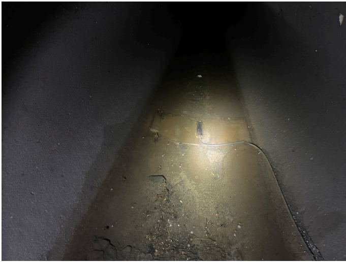
Location of flow sensor inside pipe
