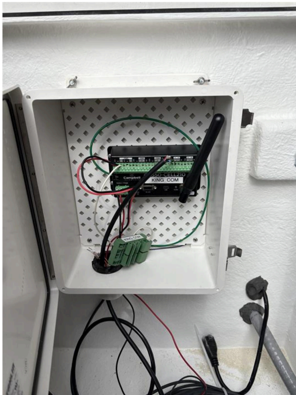
Campbell datalogger inside its enclosure
