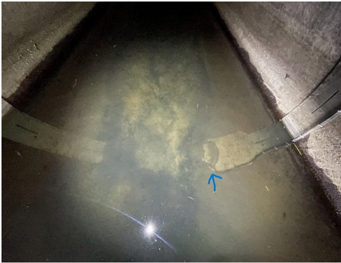
Arrow points to location of flow sensor inside the 64" pipe.
