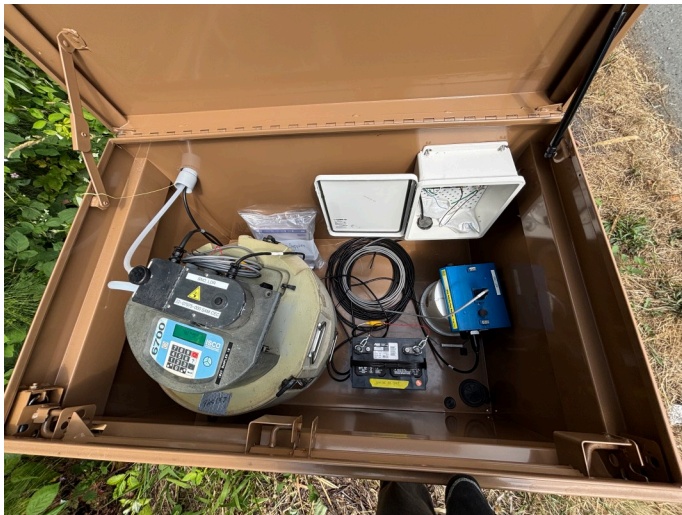
Top view of autosampler and datalogger inside knaack box structure.
