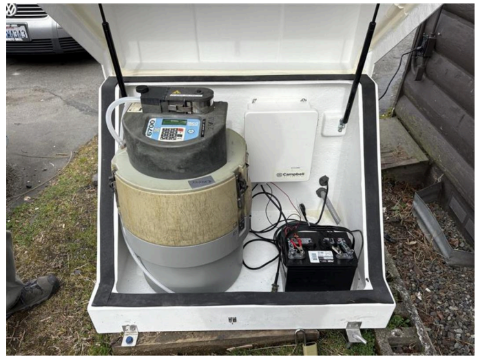
Full view of open enclosure and equipment inside which includes the ISCO autosampler, battery, and campbell datalogger enclosure
