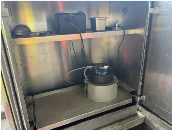
Monitoring equipment enclosure with autosampler
