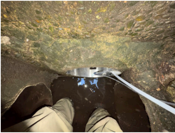
Sump photo showing birdeye of flow sensor cable and sample tubing
