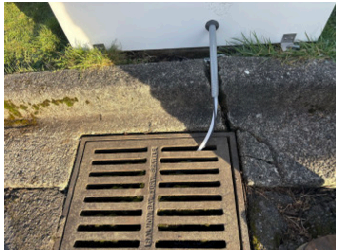
Cable/tubing from equipment enclosure to CB
