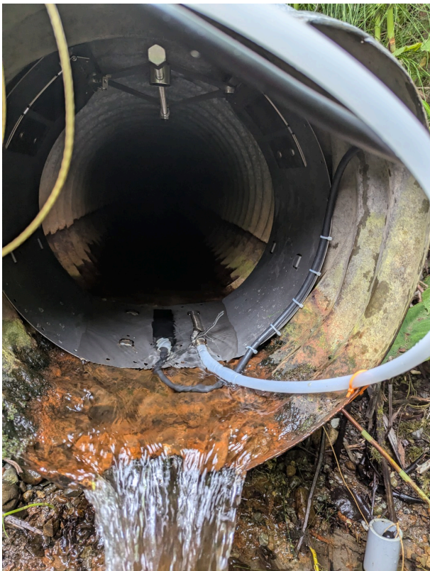
Intake tubing and flow sensor installed inside pipe
