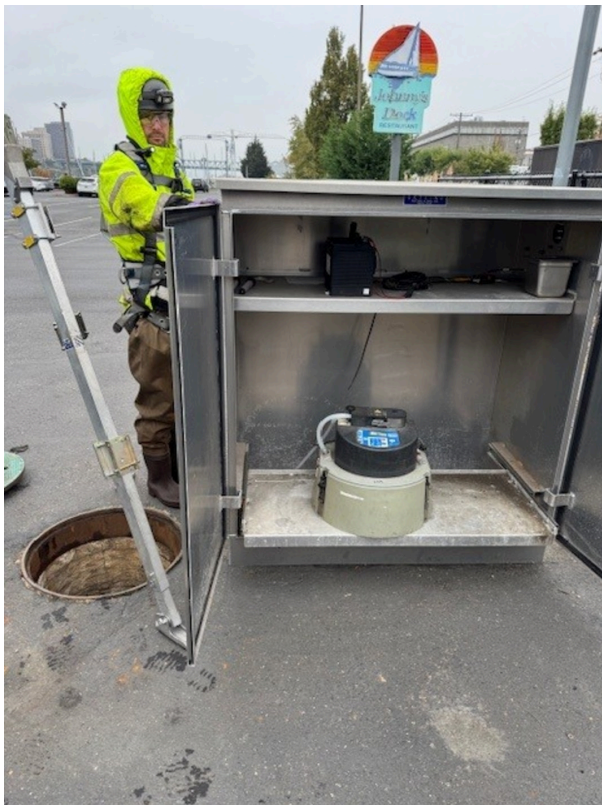
Enclosure for autosampler is located right next to the manhole access to AV sensor and intake tubing
