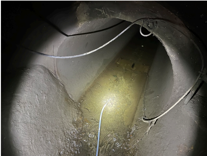
Sampler intake inside pipe relative to flow sensor
