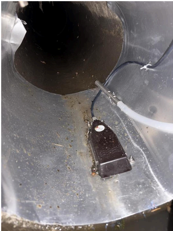
Close-up of sampler intake tubing in relation to flowmeter (facing east)
