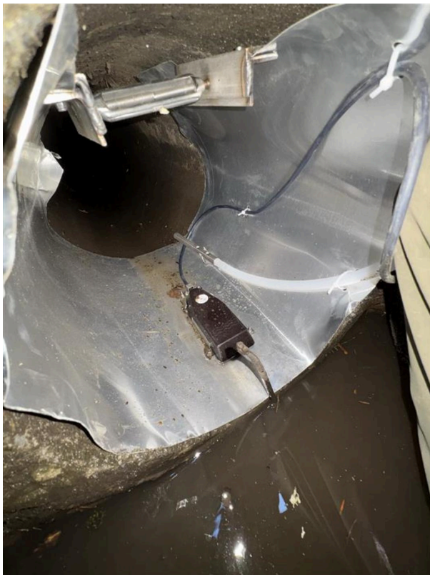
Close-up photo of flowmeter (facing East)
