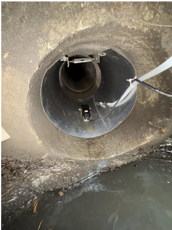
Close-up of tubing and cable connection to the intake and flowmeter inside pipe
