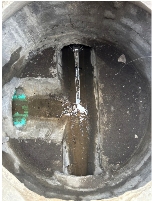
Bird-eye view of pressure transducer inside pipe
