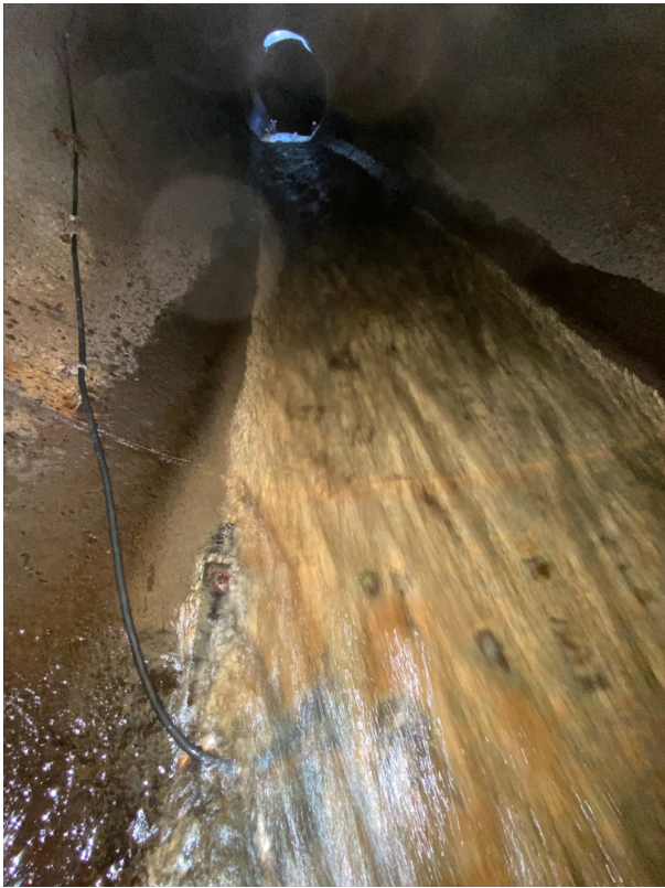
Flow sensor installed at edge of pipe
