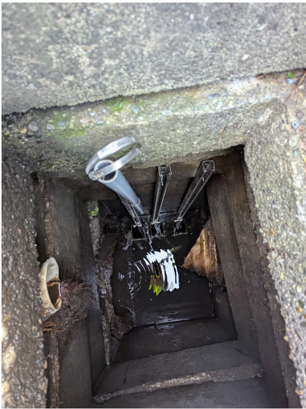
Bird-eye view of sediment traps in CB. TROLL is located inside the small conduit connected to trap installation.
