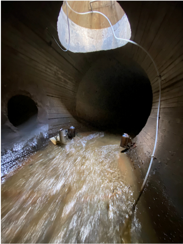
Intake tube installed on opposite side from the flow sensor
