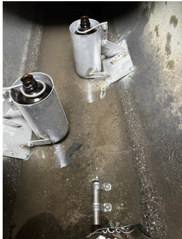
Close up of pressure transducer installation in pipe
