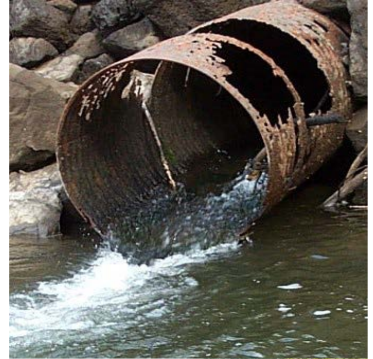
Damage or Deterioration
