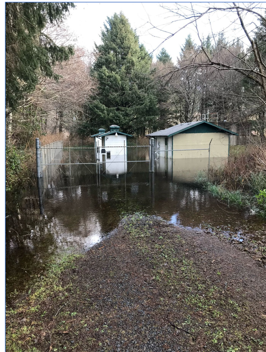
Grays Harbor County Utilities Department Water Well, 1-07-2022
